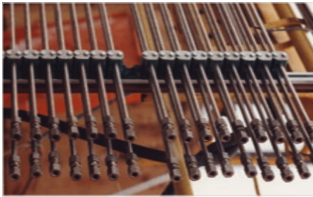
Instrumentation pipework made of stainless steel
